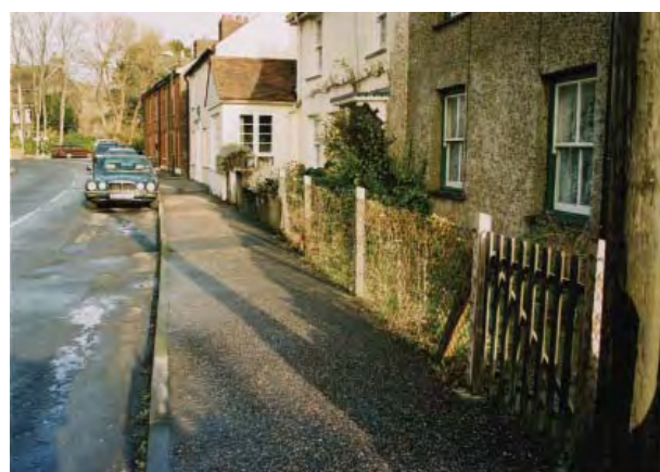
Poor quality front fence in North Street
