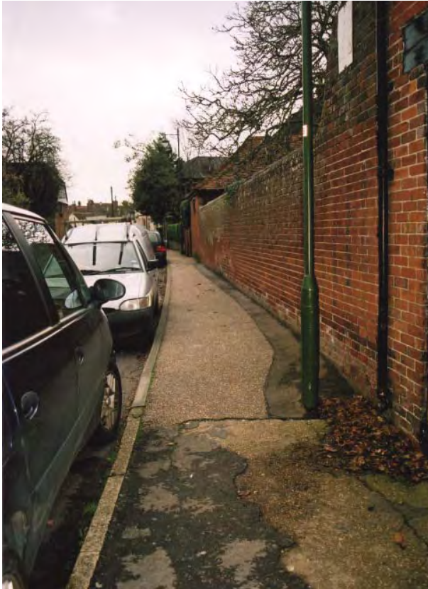
Poor quality pavements in North Street
