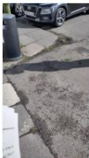
Pavement sections that need joining outside Westbourne surgery
