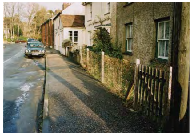
Poor quality front fence in North Street
